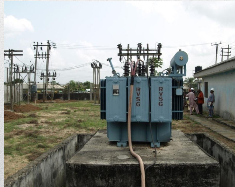
COE Injection Sub-Station to be Upgraded from 2.5 MVA to 15MVA
